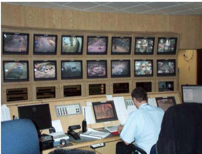
CSEL's CCTV control room
